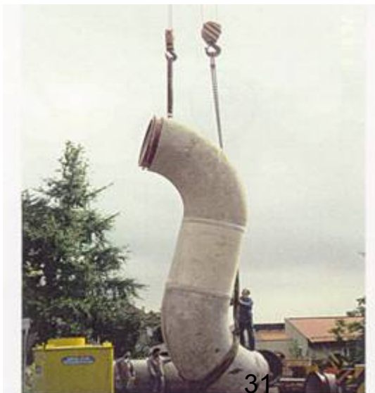
LAUSANNE (Lutry) - Station de pompage Ø 1400 mm
